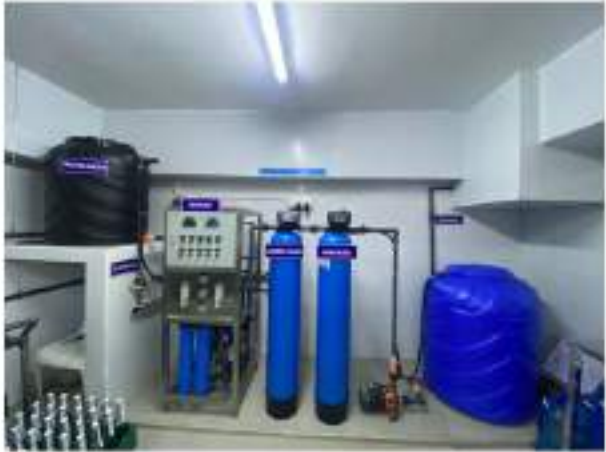
Bottling plant unit
